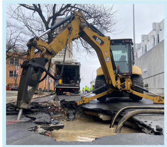
Photo 5: Water main break in Albany.
